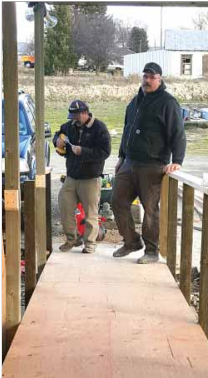
Jason Ineck (left) and Toby Robinson working on the new wheelchair ramp outside John DeOsio's home in Marsing. Photo by Mary Lou DeOsio
