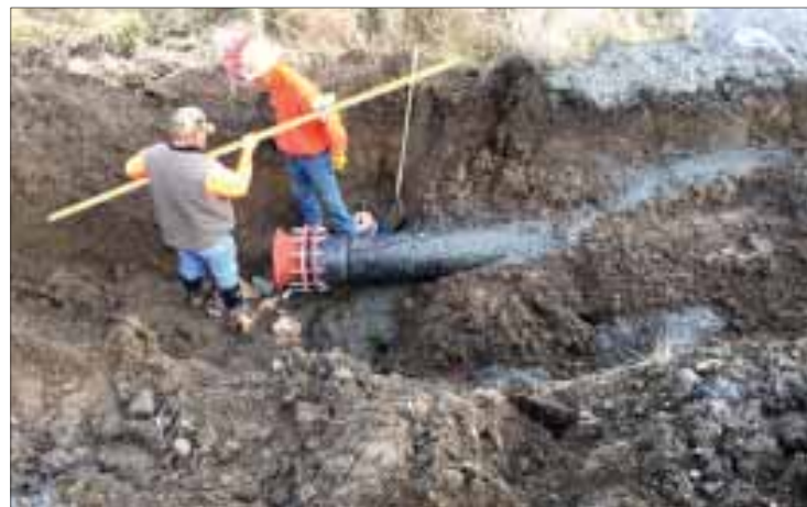
Warrington Construction crewmembers work on connecting the new 12-inch water main to the Homedale municipal system near Succor Creek. Submitted photo
