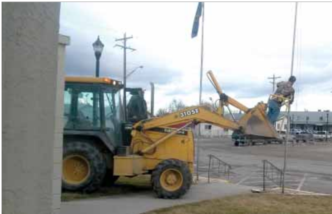
City of Homedale public works supervisor Bret Smith stands in a bucket with city maintenance worker Curtis Stansell (obscured) to repair a flagpole in front of City Hall on Thursday. City employee Jack Ulrich stands near the cab of the loader. Submitted photo
