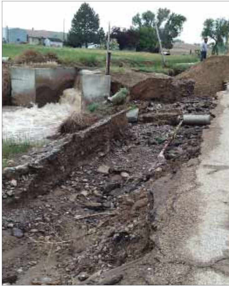
South Board of Control personnel work to clear an eroded shoulder on Gully Road on Saturday. Photo by Larry Prow
