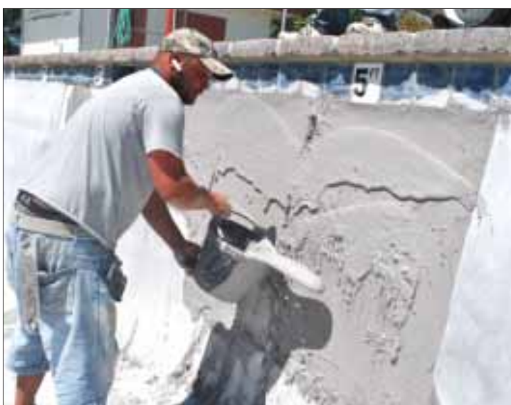
Steven Richardson, owner of Reflections Pool & Spas of Kuna, applies new plaster for repairs to Homedale's city pool May 17. Richardson said the repair work took two days to complete. He added that the color of the new plaster will fade to match the rest of the pool once it is completely cured. The pool will open for the summer upon completion of the project.
