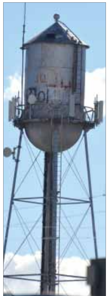
Homedale's old municipal water tank, now used as a cell tower, is getting a $10,000 facelift soon.
