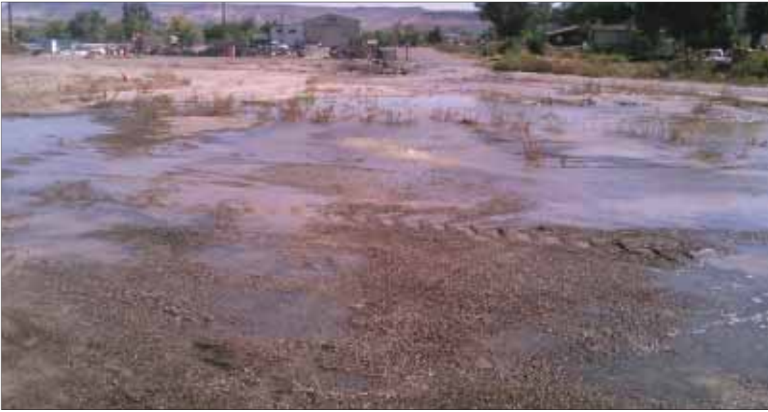
Above: Water seeps to the surface after a water main rupture in Grand View. Below: City maintenance worker Jim Burnett eyes the trench after the new pipe was installed. Submitted photos
