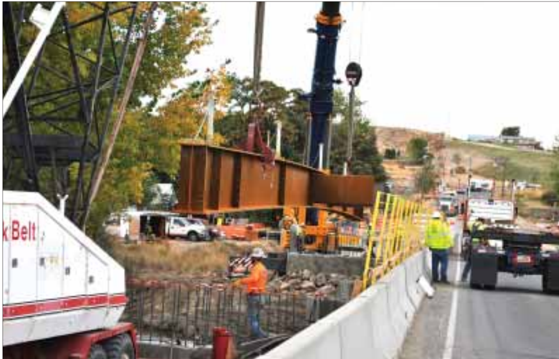
One of three steel girders is lowered into place Monday morning at the Succor Creek bridge.
