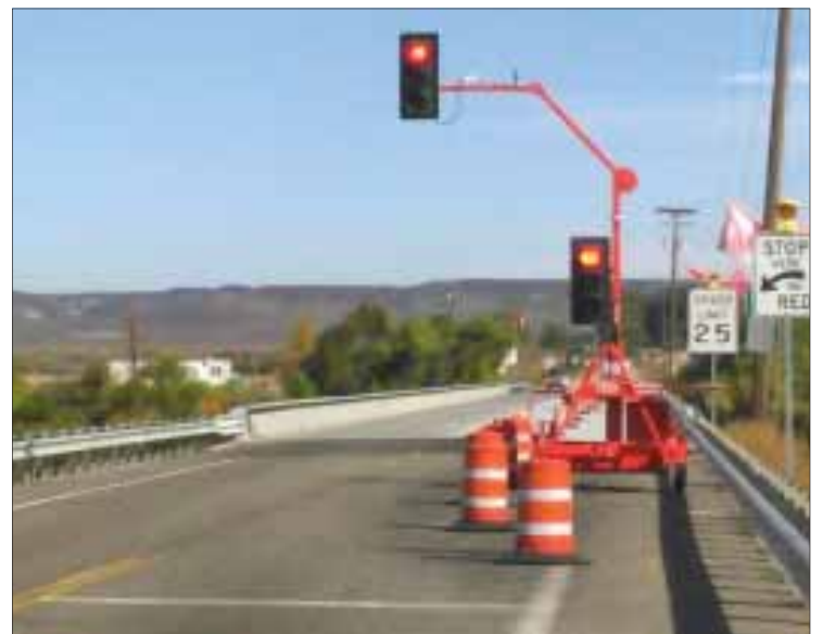
The temporary stoplight that had been regulating traffic, and aggravating Grand View-area drivers, during the Idaho highway 167 bridge project disappeared Thursday night as major construction was completed. Photo by Ed Collett
