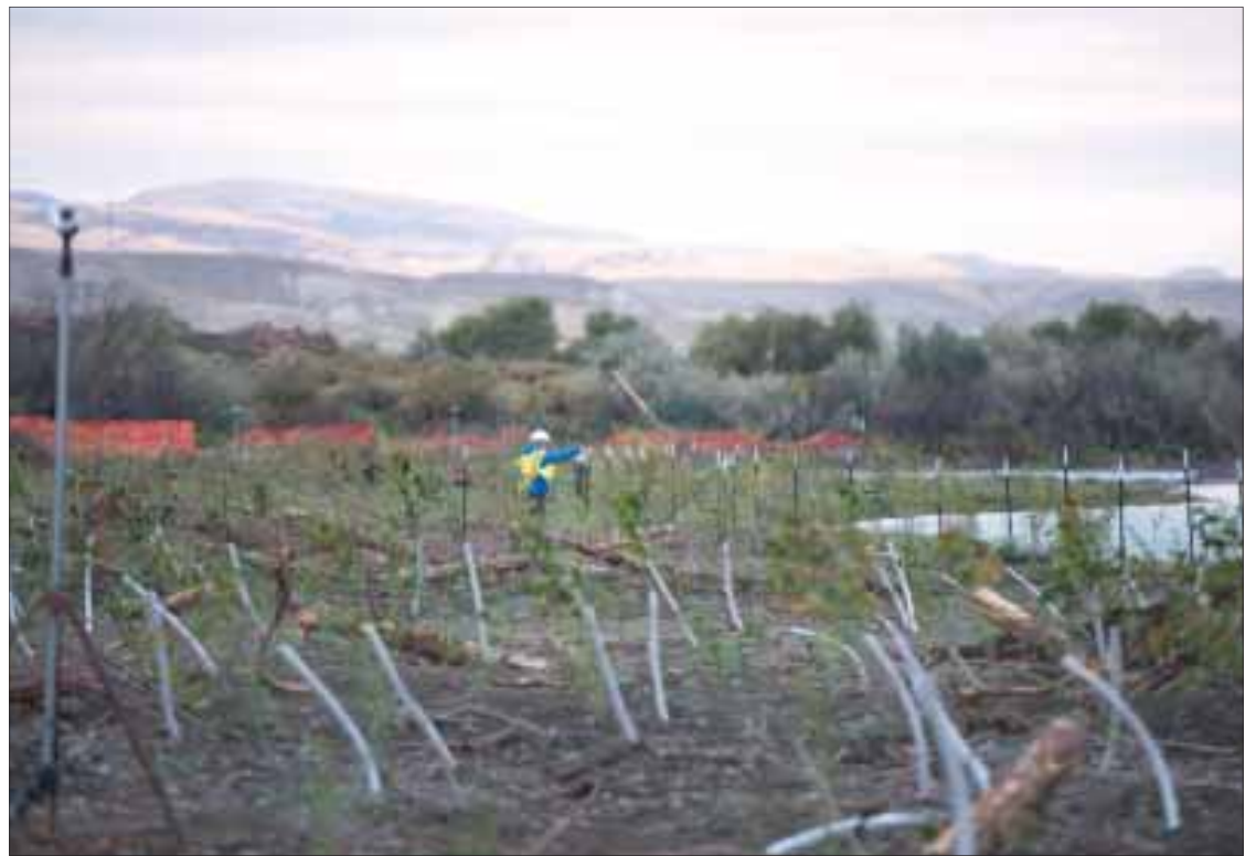
A construction crewmember checks on newly planted vegetation on expanded Bayha Island. The orange construction fencing in the background represents the island's original perimeter in the Snake River.
