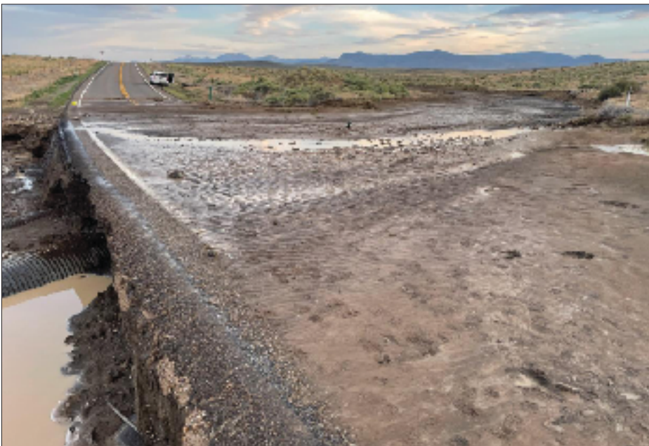
Floodwaters eroded the roadbed and put several inches of sediment on Idaho highway 78. OCSO photo
