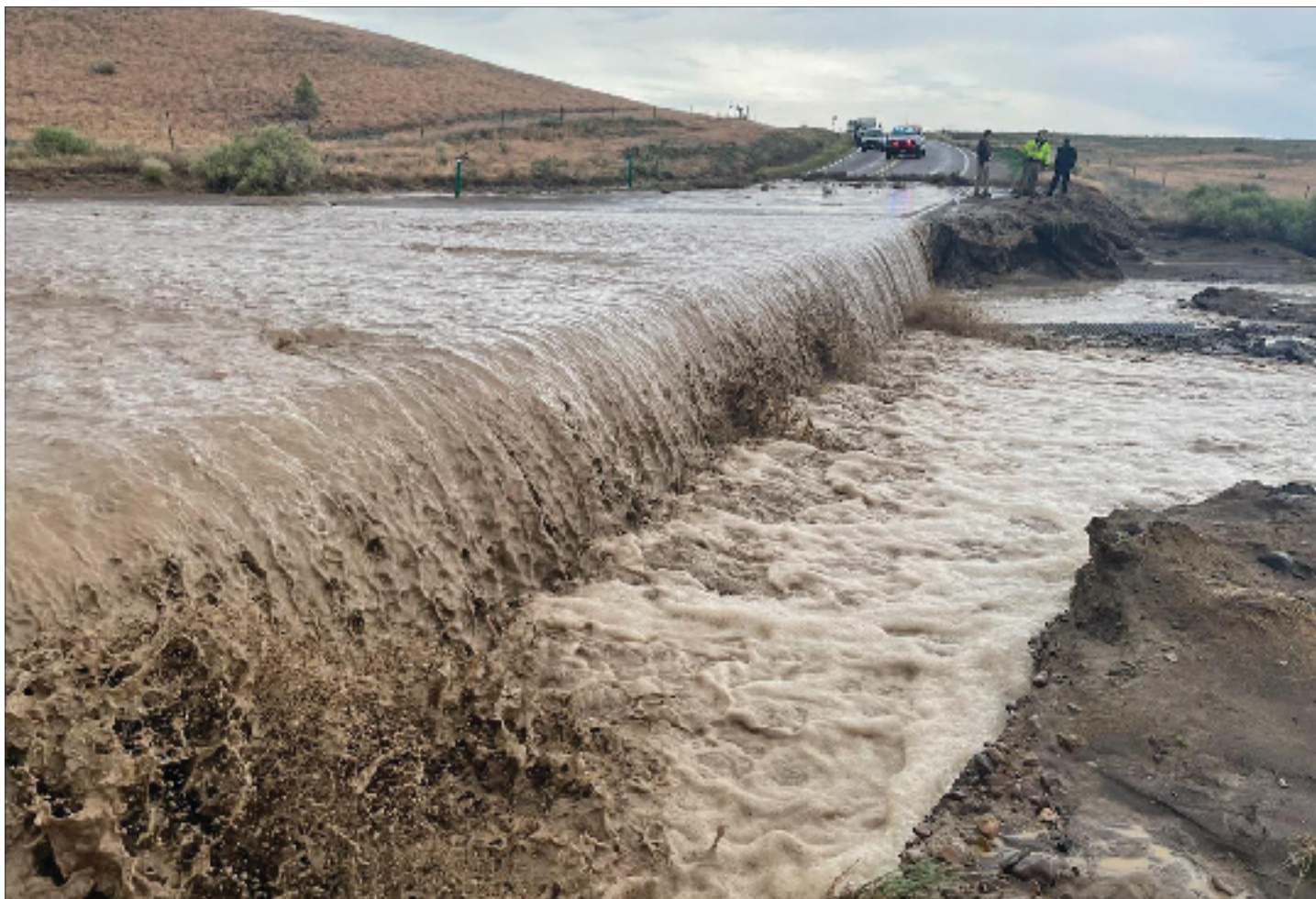
A normally dry wash ran over Idaho highway 78 on June 14, forcing closure of the Owyhee County Courthouse last Wednesday. OCSO photo
